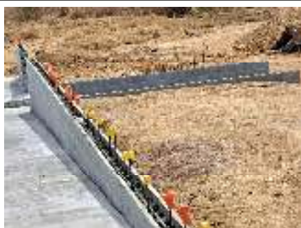
Photo 6 – Facing west to effluent collection unit
