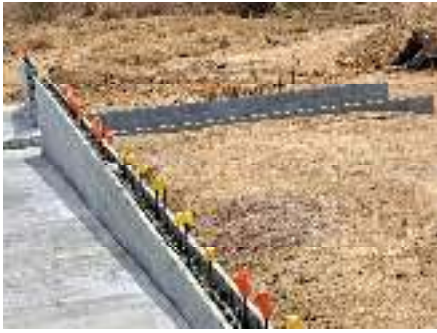
Photo 6 – Facing west to effluent collection unit
