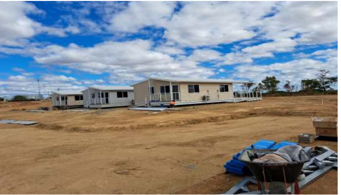
Photo 3 : Facing South East ( Houses located in the left side of the access road)
